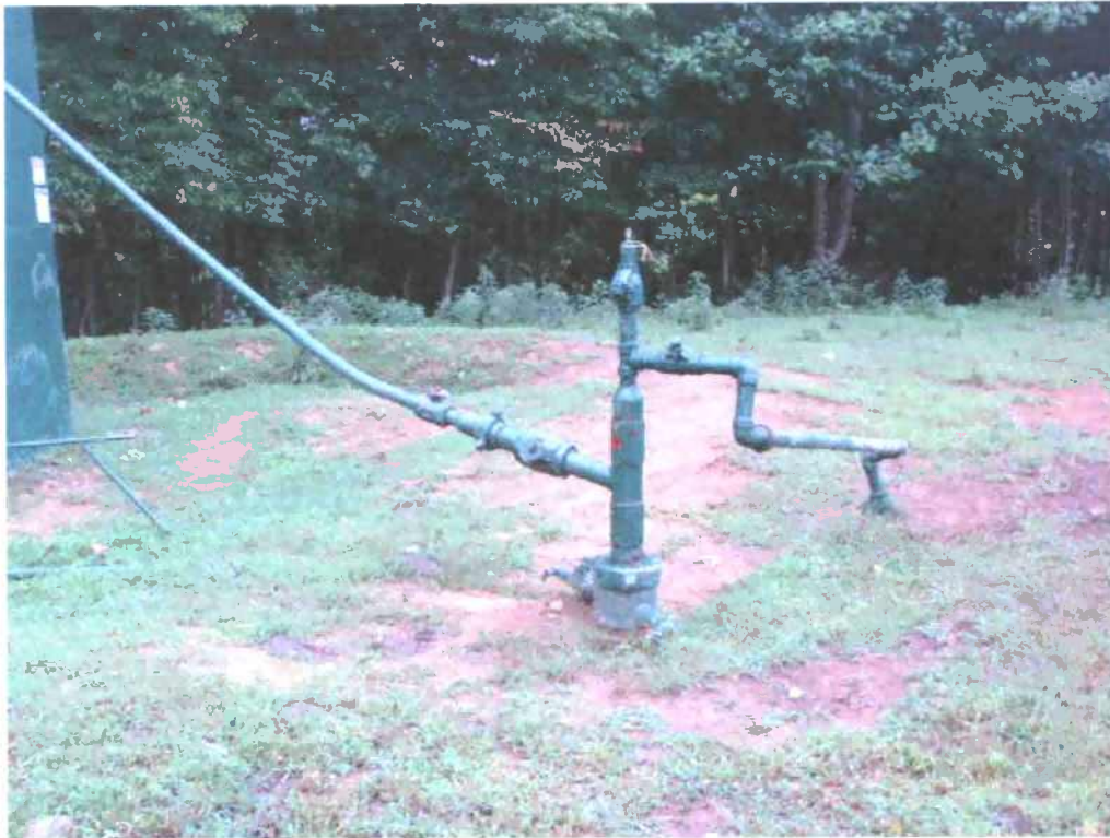
Figure 3. Keyspan well located 2,800 feet north-northwest of 6:26:35 a.m. Vaisala lightning strike location that shattered a large tree. Well is serviced by an approximate 3-inch diameter metal pipe that is buried until exposed at a monitoring station 300 feet to the northeast. No evidence of lightning damage was apparent to the metal, or the surrounding trees and ground.
